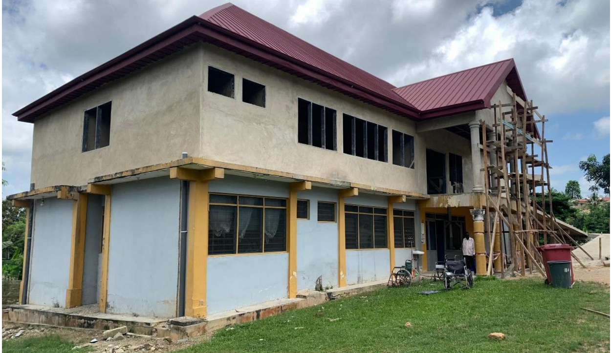
1No. Health Center with male ward, female ward, Nurses Station, Dispensary, Consulting Room, Staff Washroom at Daboase (Phase II)
