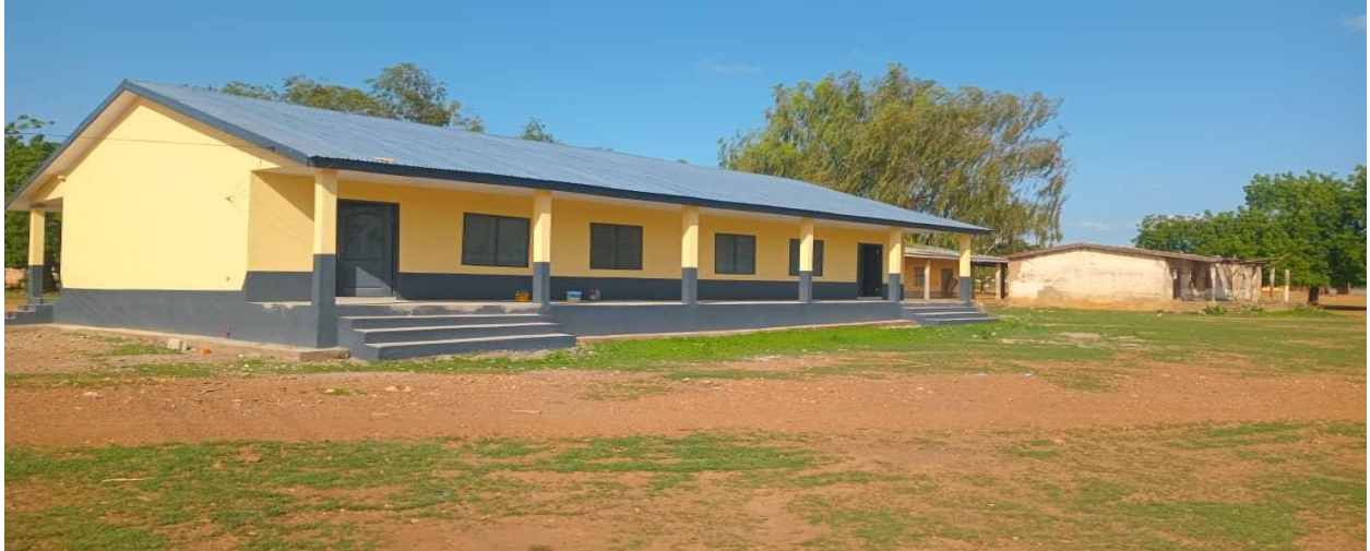
Rehabilitated 2-Unit Kongo Kg Block and Rehabilitation of 2-Unit Classroom Block At Kongo for CNC-SOCO
