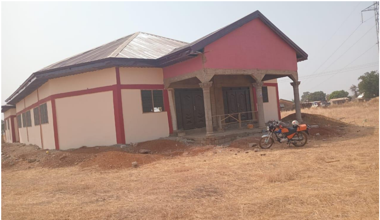
Completed community center with a hall, store, an office and 1No 3unit bath and toilet at Asonge 70% Completed-SOCO.
