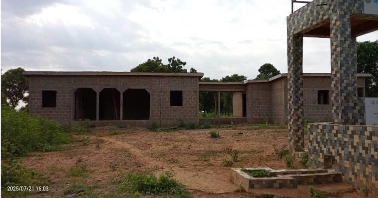
Construction of 1 No. Community-Based Health Planning and Services (CHPS) Compound at Singa -Ongoing
