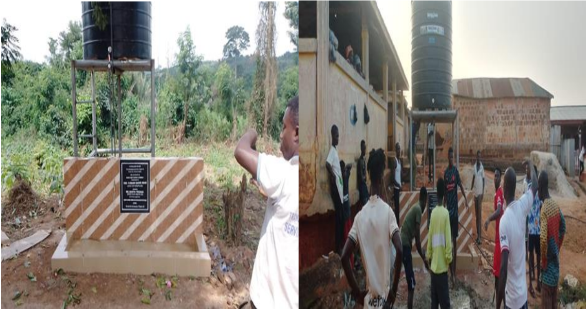
Figure 3: Completed a mechanized Bole hole with poly tank and electricity connection at Gomoa Ajumako
