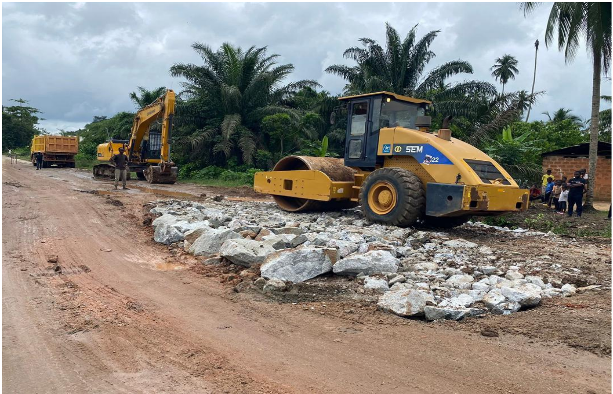
Dredging, filling and compacting of the Assin Kyekyewere highway culvert and drains
