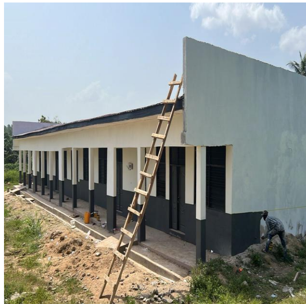
Completed the construction of 1 No 3unit Classroom Block with office and store at Fiahwia
