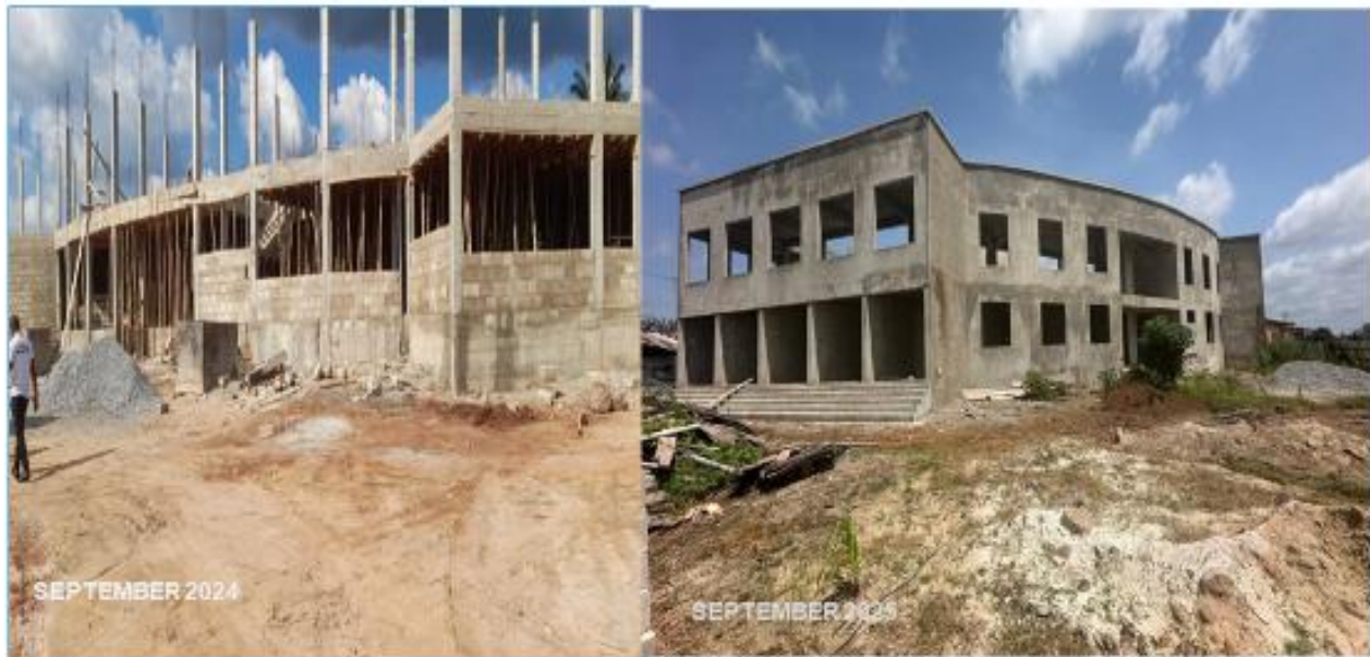
Picture 2: Completed 1no. 2-storey conference hall with offices and lockable shop at Berekum (GSCSP)
