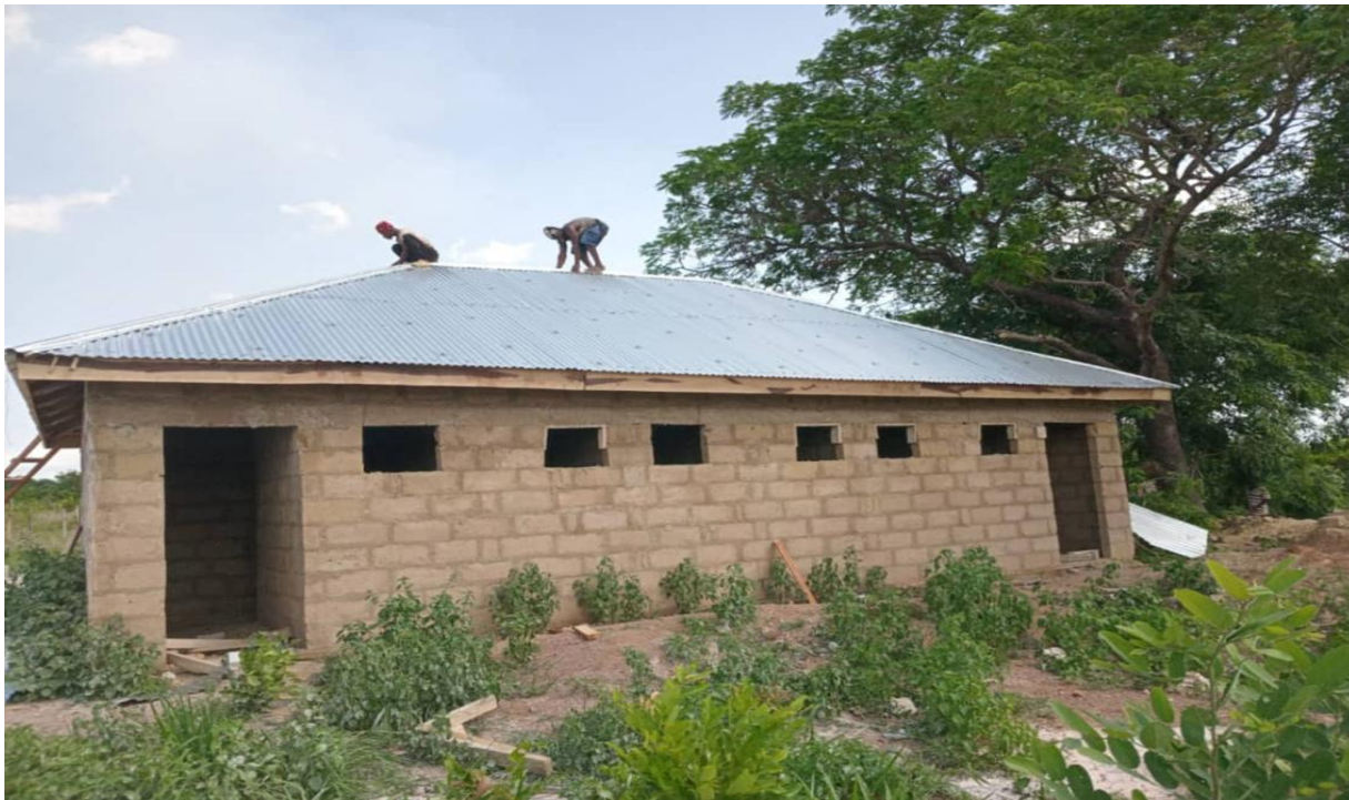
Picture 5: Constructed 1no. 12-Seater W/C Toilet with Mechanized Borehole at Bongase Fish Market
