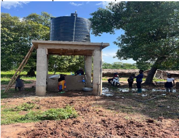
Drilled and Mechanized 1No Borehole at Bonkro (Remark: completed and in use)
