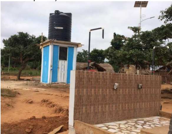
Drilled and Mechanized 1No Borehole at Kyerefene (Remark: completed and in use)
