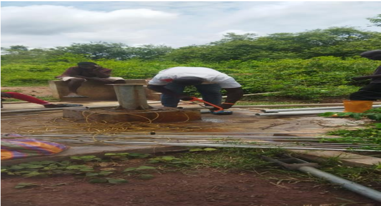
Drilling of 3No. Boreholes fitted with hand-pumps at Abotantri, Mossi Panin and Offei
