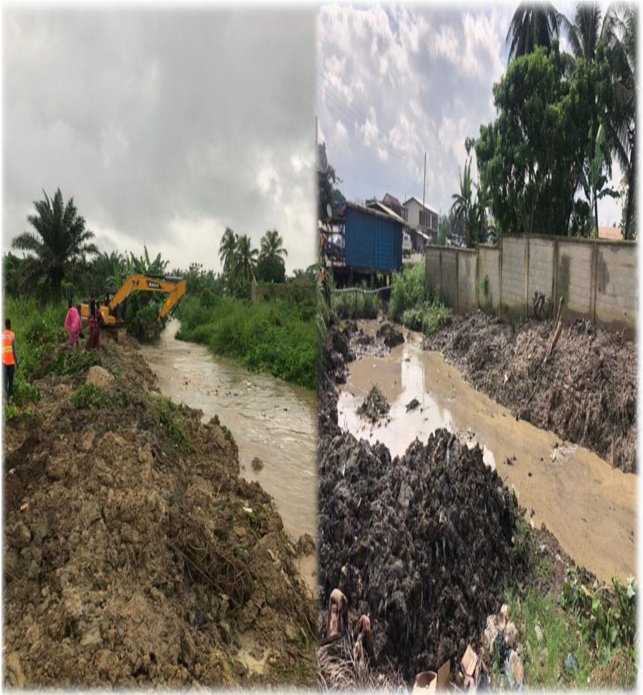
Dregded Agona SDA - Stadium road storm drain and Hopes and Dreams - Baidoo Bonso SHS storm drain
