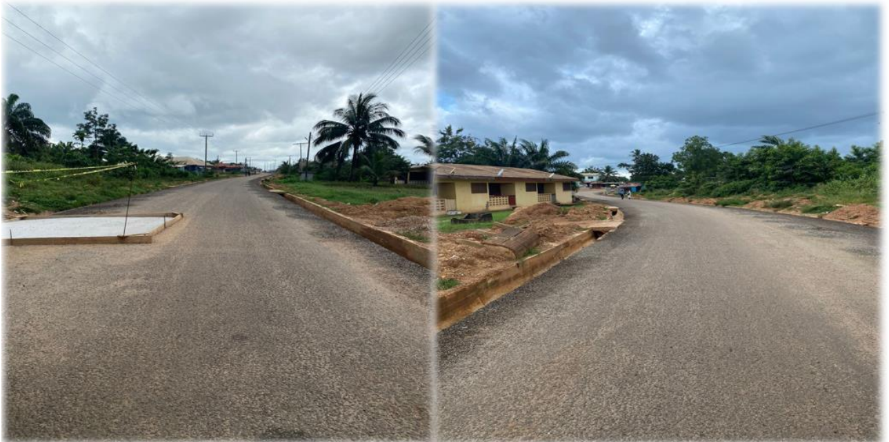
Construction of Double Seal Bituminous Road with Side Drains, 3No. Pipe Culvert and 1No. Box Culvert – 0.6km of Road at Damtse
