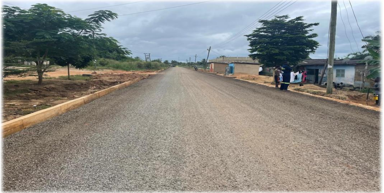
Construction of Double Seal Bituminous Road with Side Drains, 3No. Pipe Culvert and 2No. Box Culvert – 1.5km of Road at Domeabra
