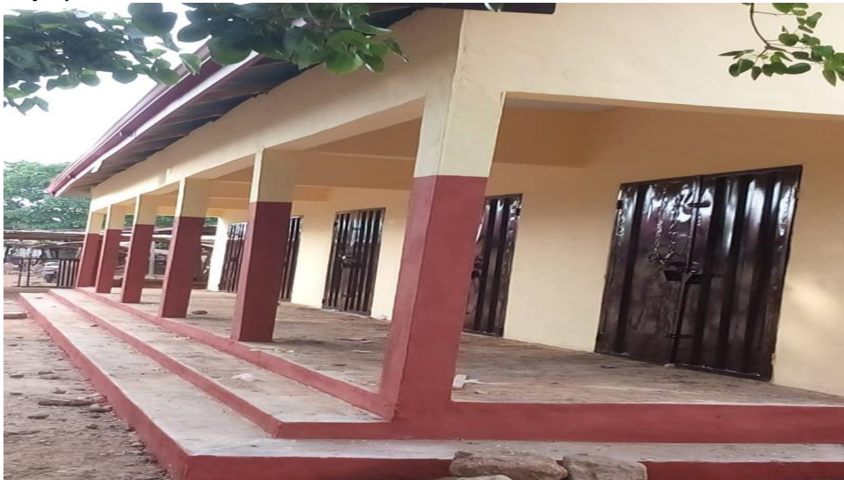
Construction of 2 no. 16 unit Stalls and 2 no. 5 unit Lockable Stores at Bussie and Kojokperi Markets
