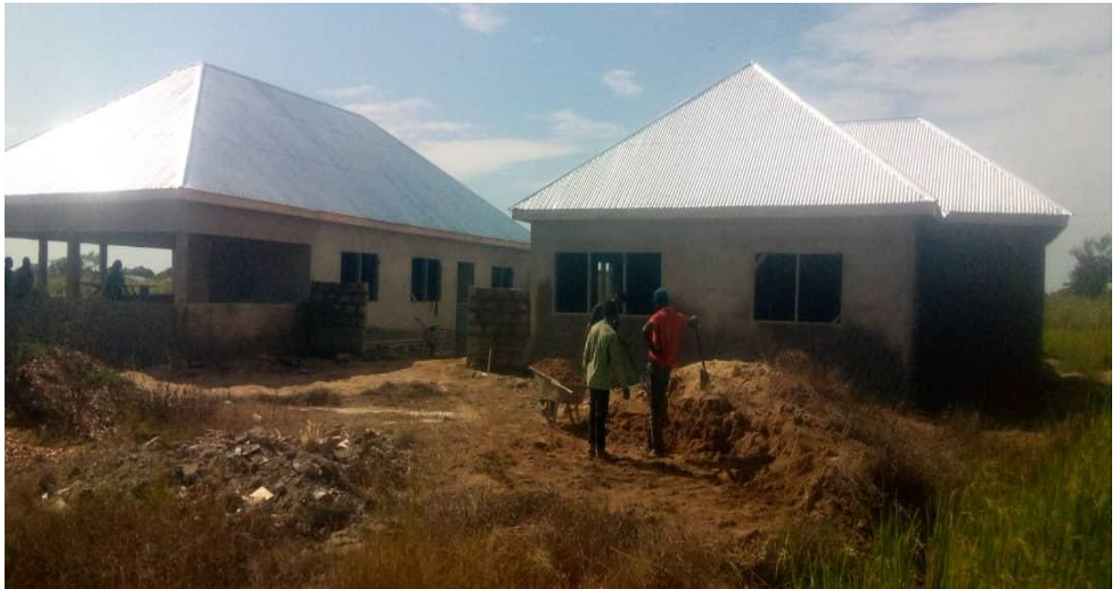
Completion of 1no. CHPS compound with urinal, KVIP toilet and furnishing Yimonsa under SOCO
