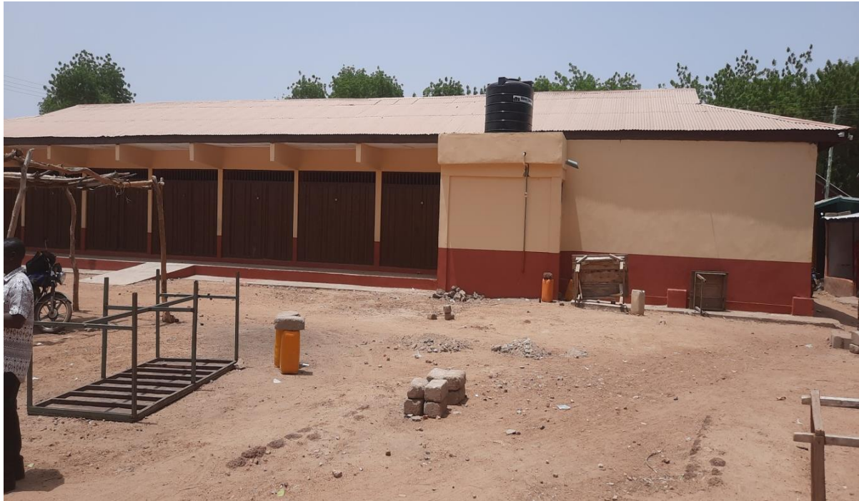
Completed 65-unit lockable stores and 2no. Urinals at the new Sandema market under SOCO
