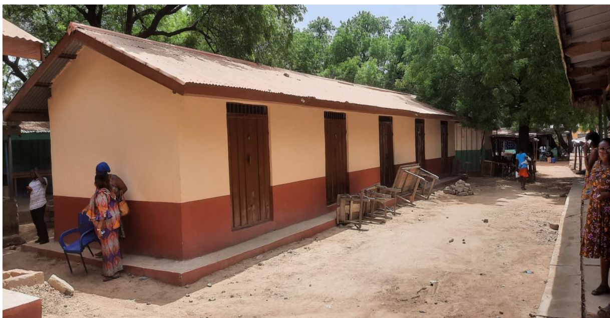
Rehabilitated 1no. 15-unit lockable stores at the old Sandema market under SOCO
