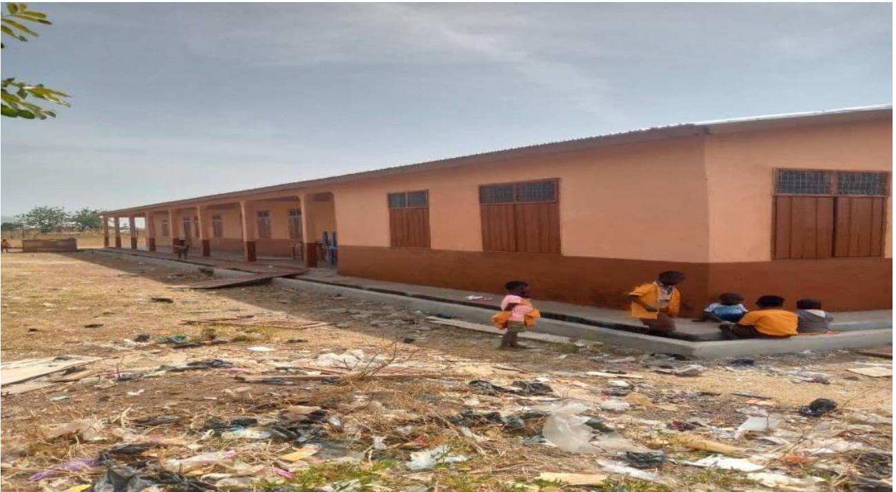
Construction of 1No. 2 Unit Classroom Block with office and store at Yalugu
