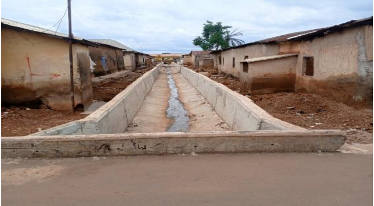
Figure 2: U-Drain at Kumfong
