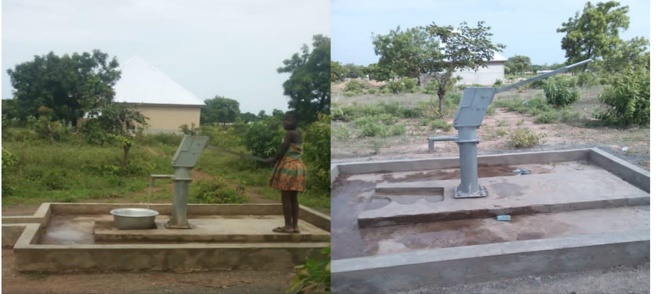
DRILLING AND INSTALLATION OF 1NO. BOREHOLE AT NKPANGINI CHPS COMPOUND (COMPLETED) BY SOCO
