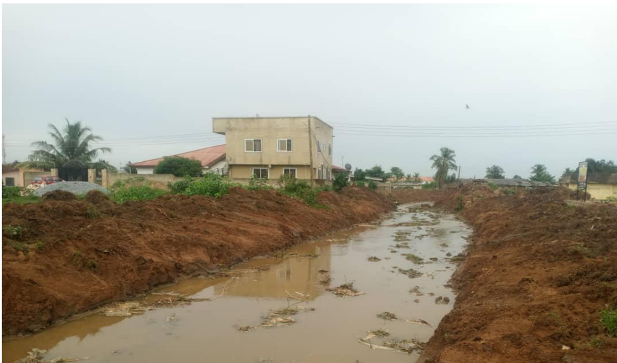
Dredging Works at Lane 5 Down, Anti-Aku, Dredging of 280m Stream at Vicolis and Dredging of 310m Stream at Olebu
