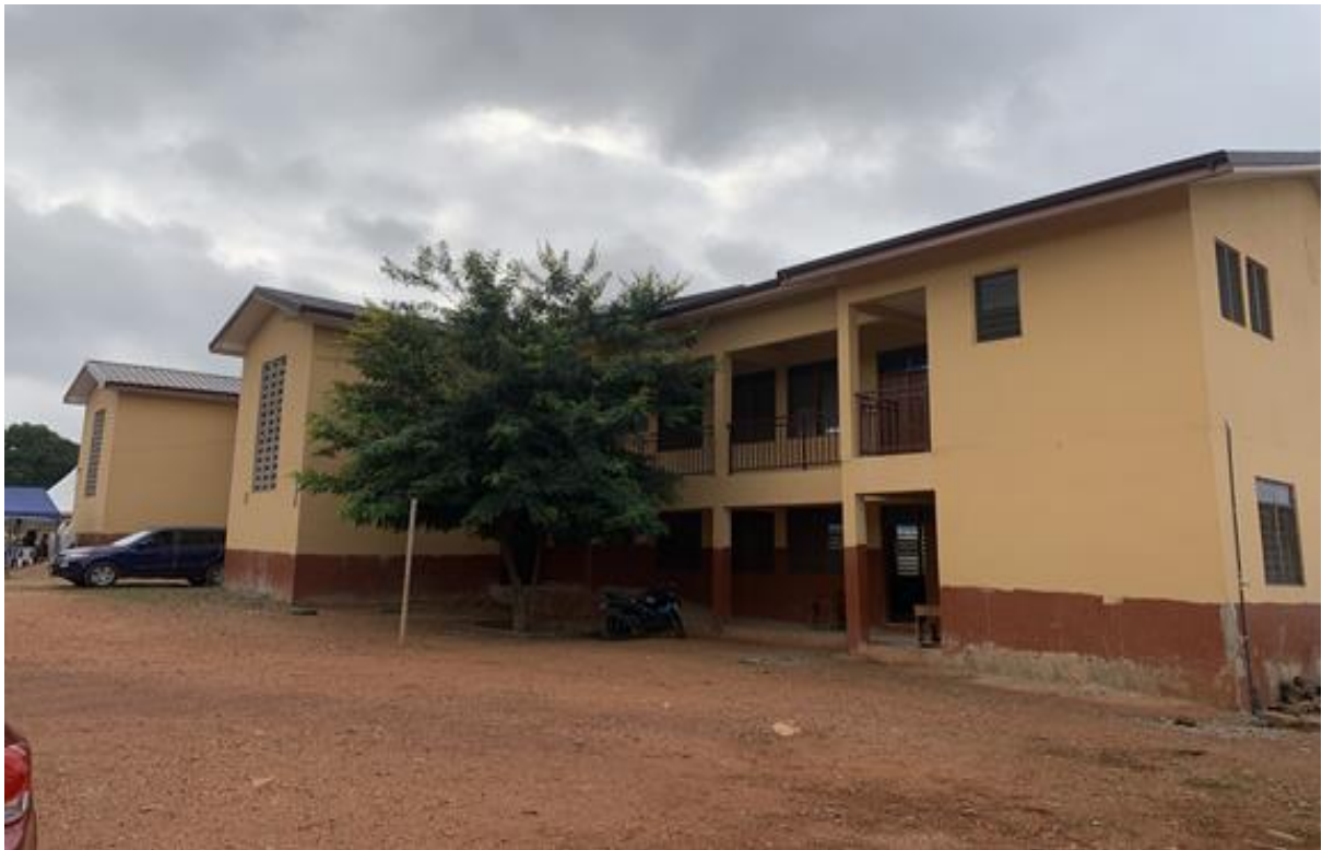
Constructed 6- unit Classroom Block with ancillary's facilities at Abelenkpe Basic School (Phase 2)
