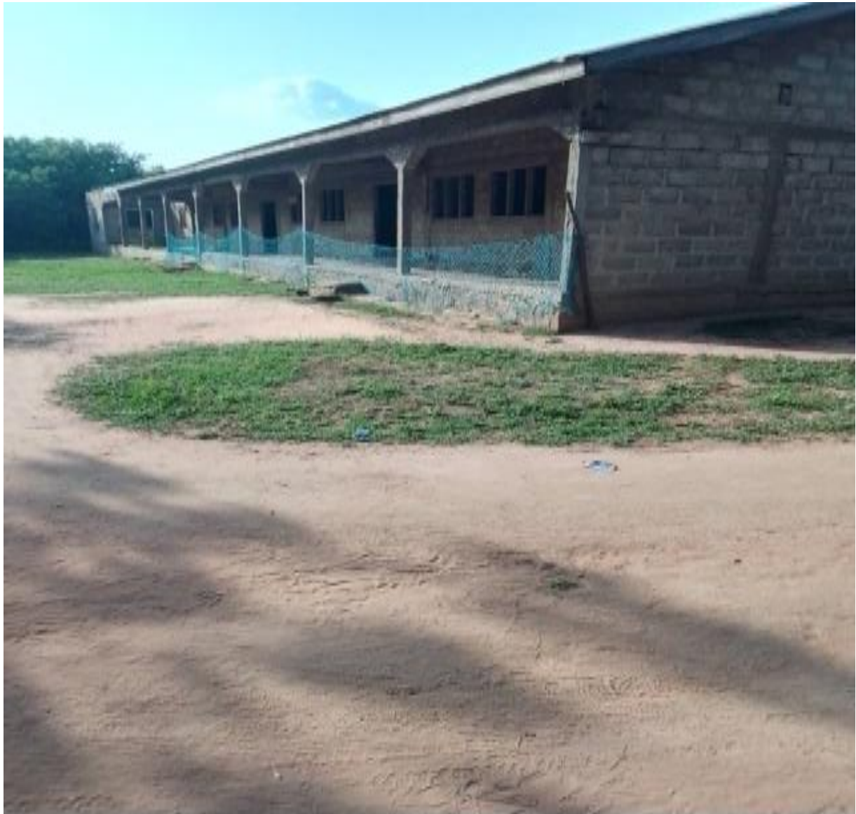
Fig 9: Construction of 3-Unit classroom block for basic school at Sihu Norfegali (75% Complete)
