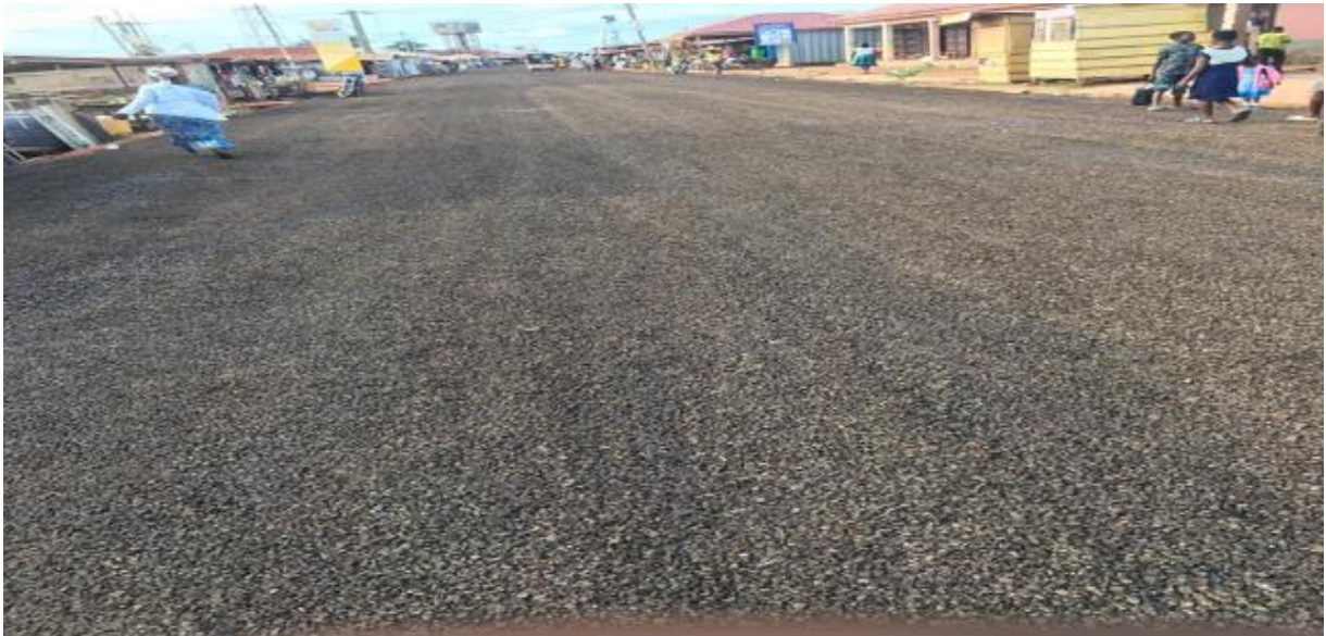
Fig 6: Construction of Bituminous Surfacing of 0.8km GCB Bank Roads At Donkorkrom (65% Complete)
