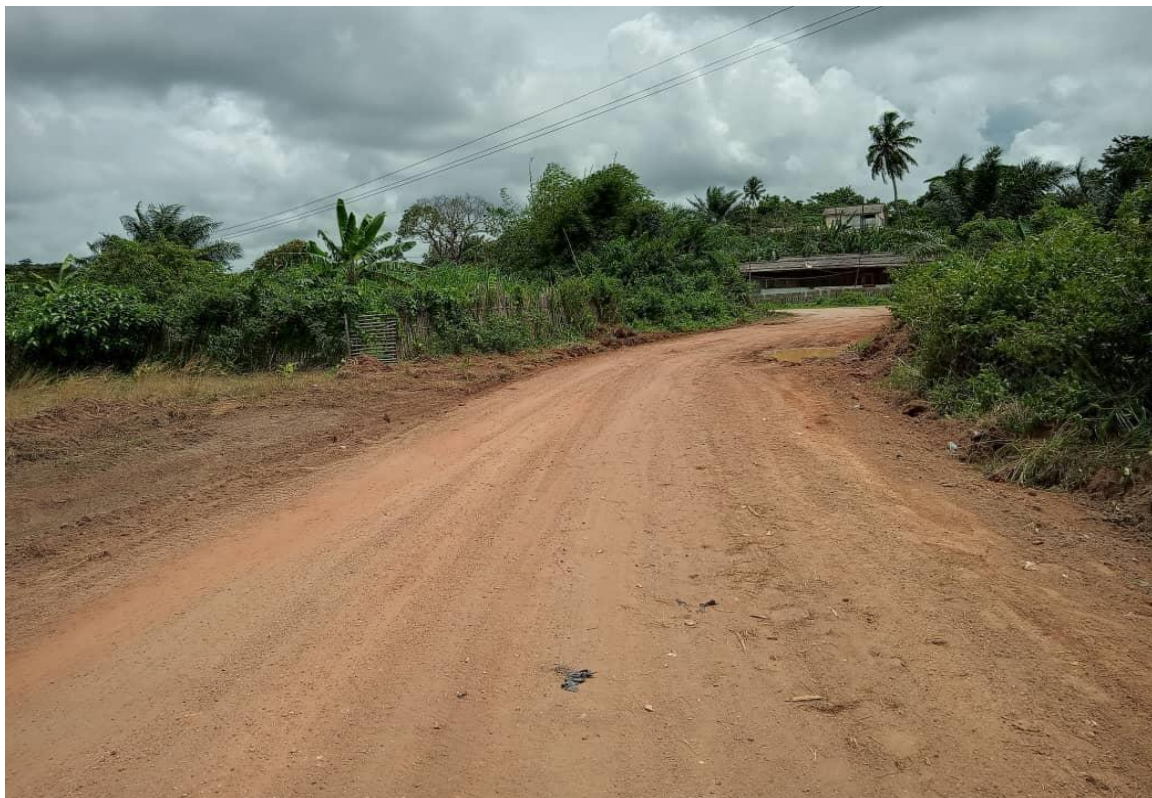
Construction of 1.5km Road at Abura Dunkwa, 130m Road At Tetsi, 280m Road
