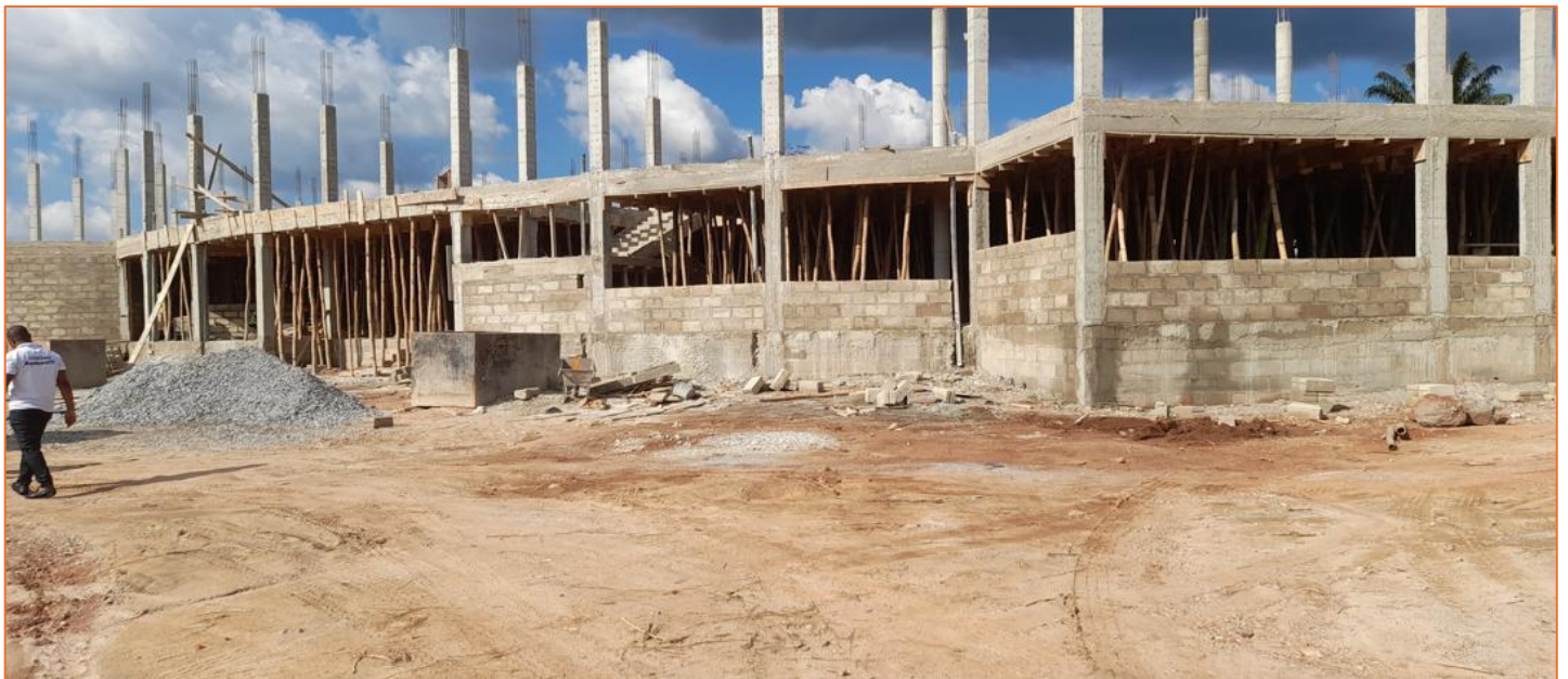
Constructed of 1no. 2-storey conference hall with offices and lockable shop at Berekum.
