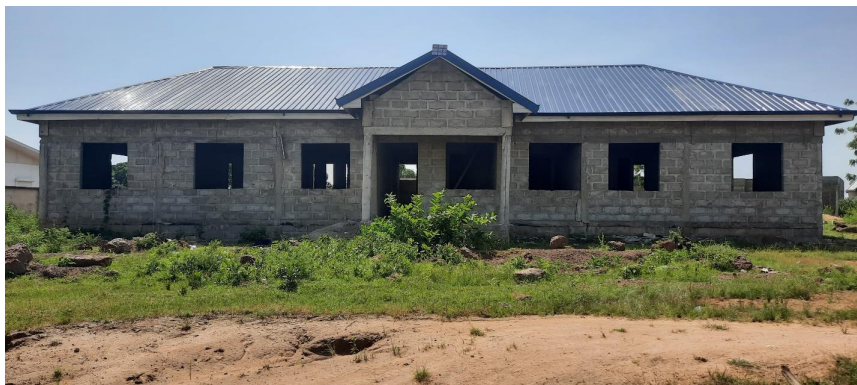
Constructed 1No. disability friendly District Health Administration office block with ancillary facilities at Garu (DACF-RFG)
