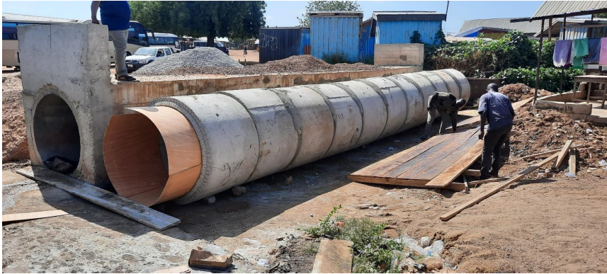
Constructed Ino. Box Culverts to link the Garu Central Lorry Park to the Small Ruminants market at Garu (DACF-RFG)
