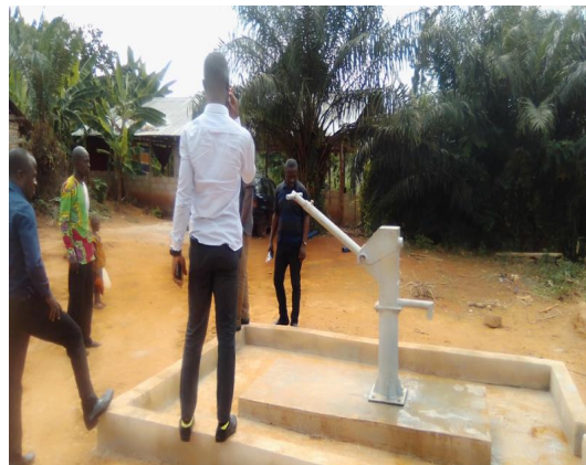
3 NO. HAND PUMP BOREHOLES, LOCATION: TERCHIRE, BEDOME, ADIESUA
