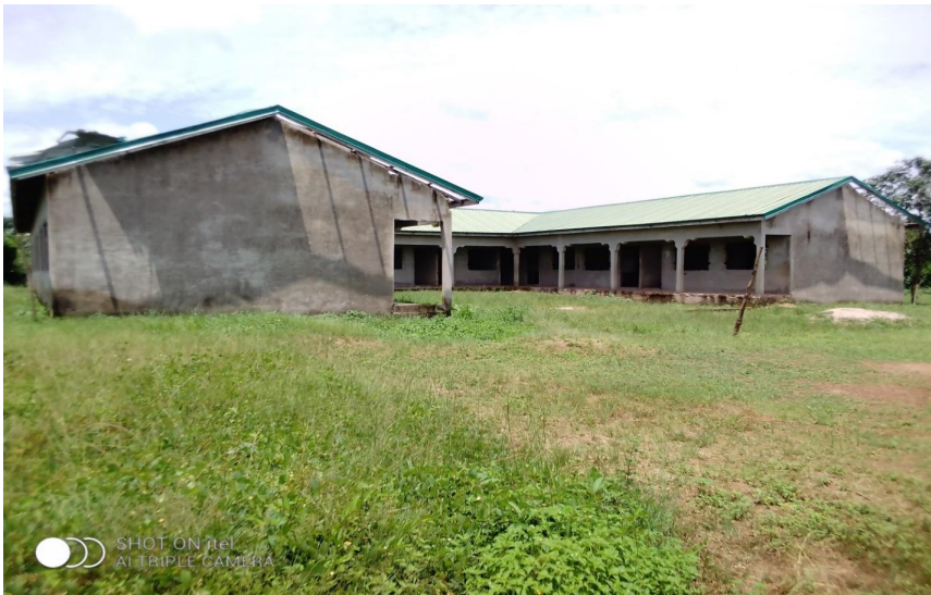
Construction of 1No.6-Unit Classroom Block, Office, Store, Computer laboratory and Staff Common Room with 1No. 4-Seater KVIP Toilet at Mankesim Primary (DACF Project)
