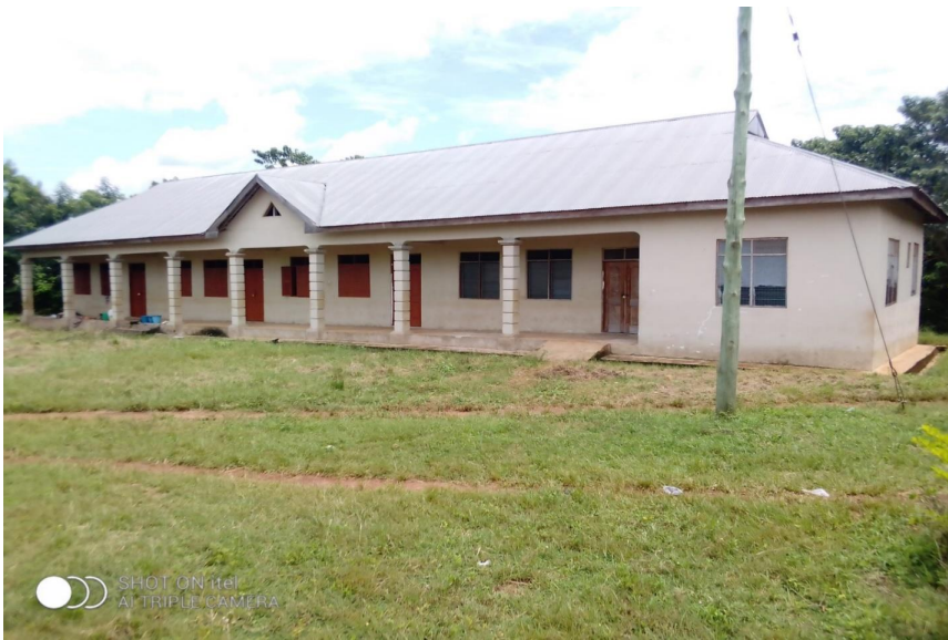
Construction of 1No. 3-Unit Classroom Block with Office, Store, Computer Lab and 2-Seater Toilet Facility at Mehame (DACF Project)
