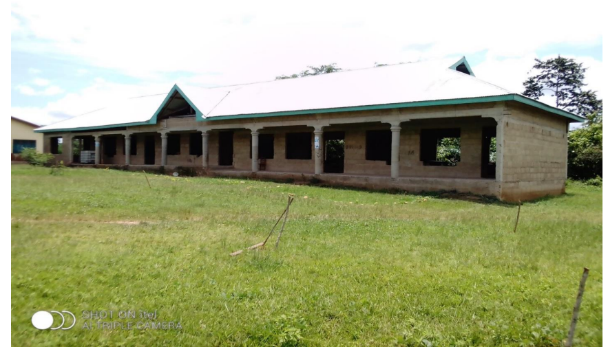
Construction of 1No. 3-Unit Classroom Block with Office, Store and 2-Seater Toilet Facility at KwakuNyumah (DACF Project)
