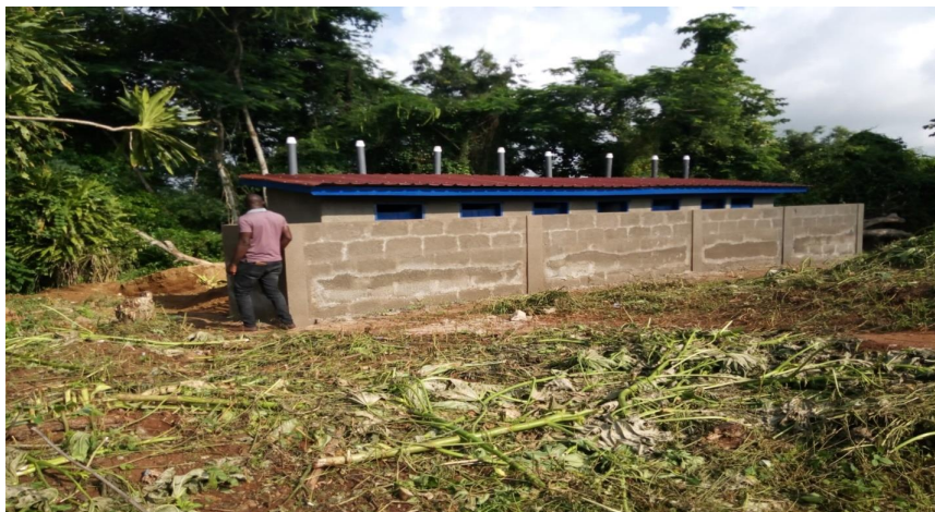
6 Seater Sanitary Facility
