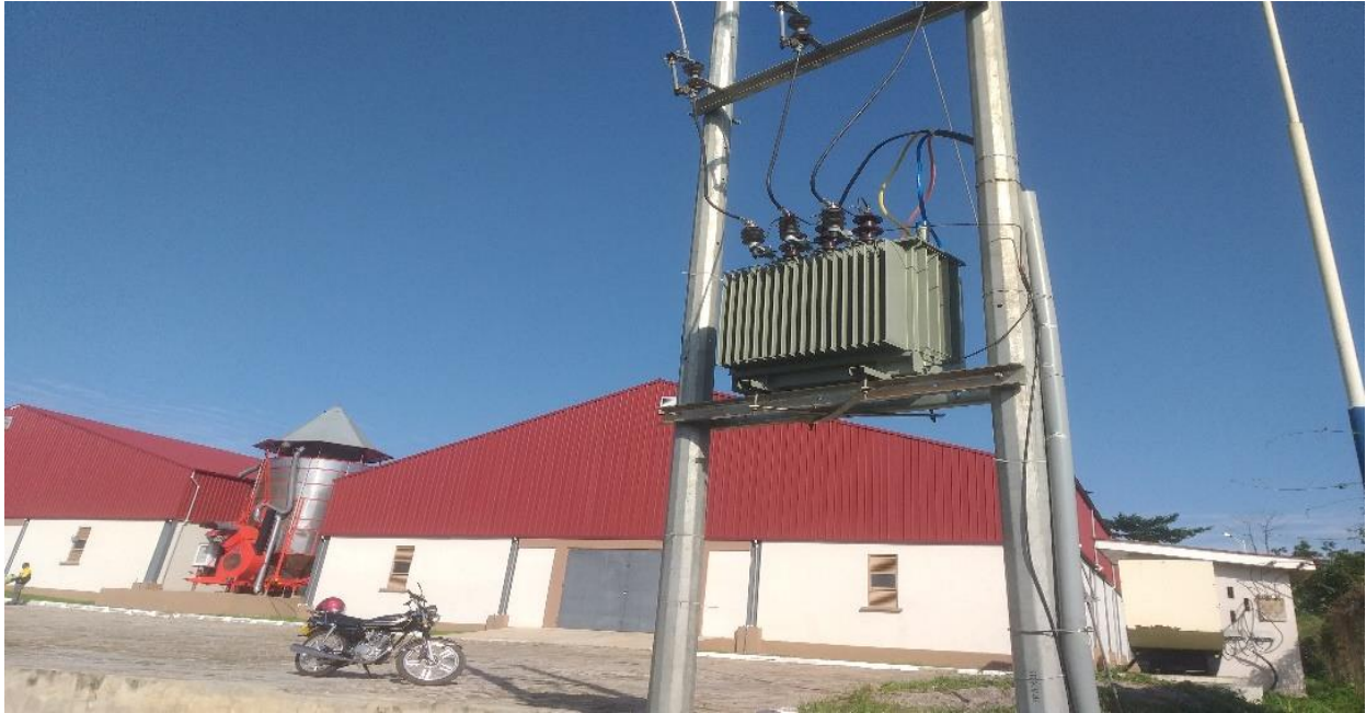
Figure 7: Installation of Transformer for Maize Processing Factory (1DIF) and Connection to the National Grade –DACF
