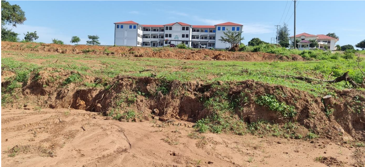
Figure 15: Clearing and Earth work at the forecourt of the District administration block for recreation facility
